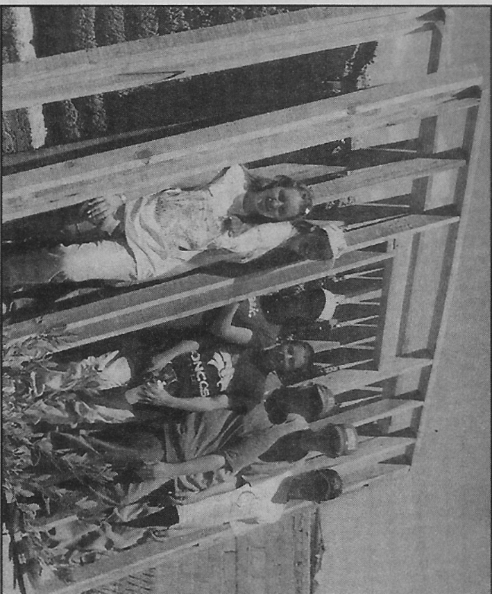
"Putting up the walls." Builders from St. Mary Magdalene, Boulder, pose during construction of a home in Juárez, Chihuahua.
